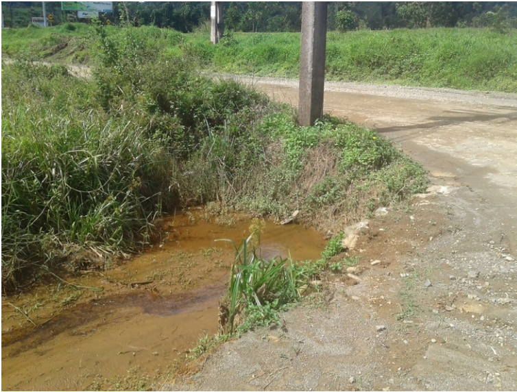
FIG. 14.2 A blocked drainage system in Wainadoi. Source: Picture was taken by S. Liligeto in 2018. No permission required.
