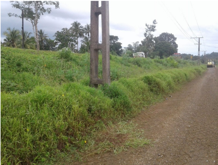
FIG. 14.3 The elevated Queen's Highway. The elevated road causes backflow of water and blockage of natural drainage outlets. Source: Picture was taken by S. Liligeto in 2018. No permission required.
