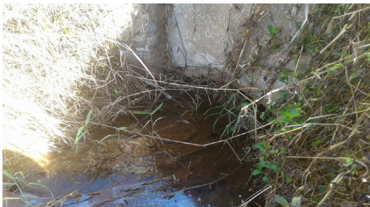
FIG. 14.4 A blocked drainage system in Navua. Source: Picture was taken by S. Liligeto in 2018. No permission required.
